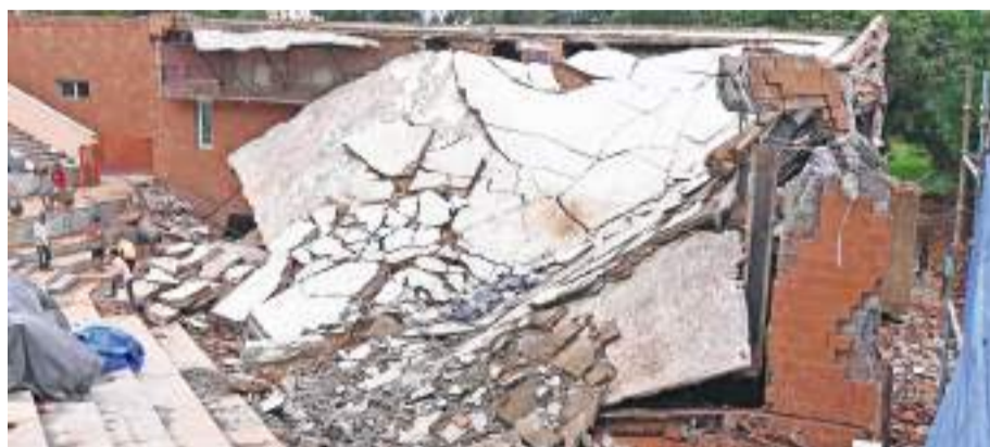
ALL FALL DOWN: The entire slab of the open auditorium that collapsed in the late hours of Sunday.
