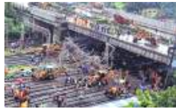
Hence, there will be some delay in opening one arm of the bridge," said a senior civic official. The work
